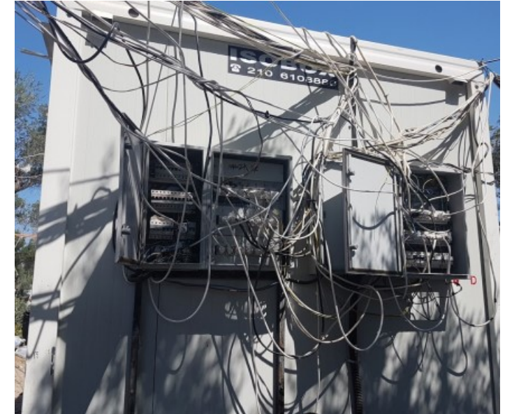
A maze of electrical connections running to tents
