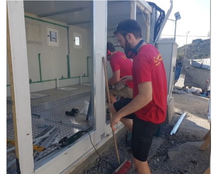
Refurbishing a toilet container after completely gutting the interior of the previously unusable facility
