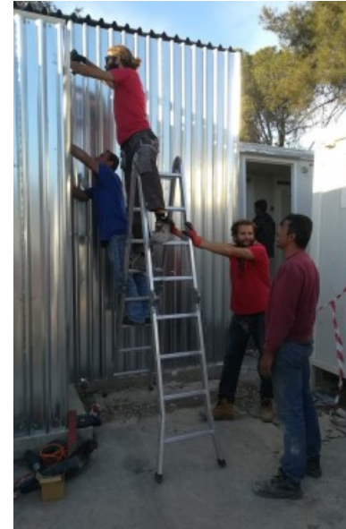
Building a structure to house the boiler which heats water in the shower block
