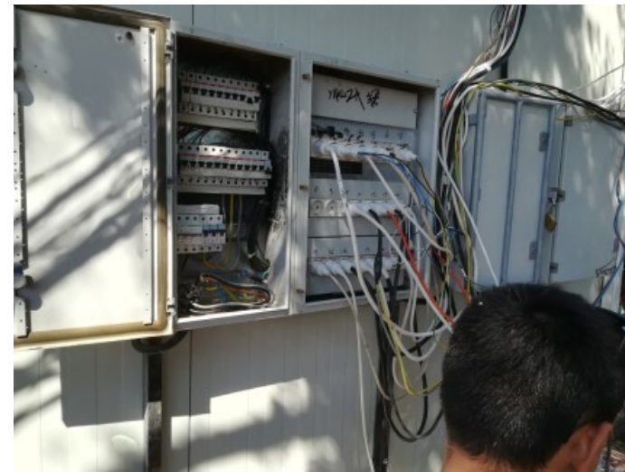
A newly-installed electrical box
